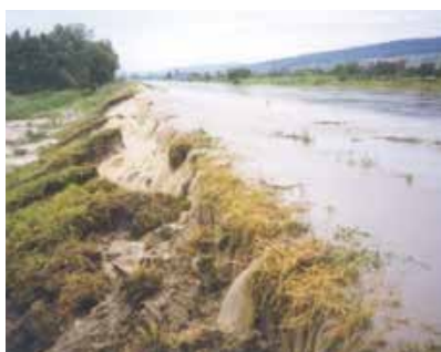
Šúrsky canal left bank dike overtopping in 1999
