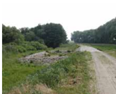
Outlet (intake) object in the dike of Šúrsky canal
